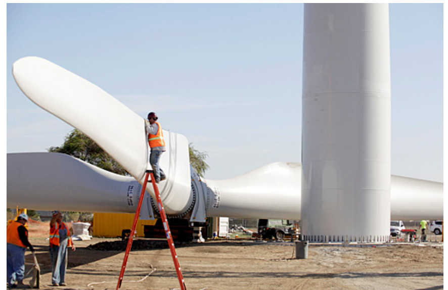
Installation of the wind turbine at the Anheuser-Busch brewery (Source: Daily Republic)
